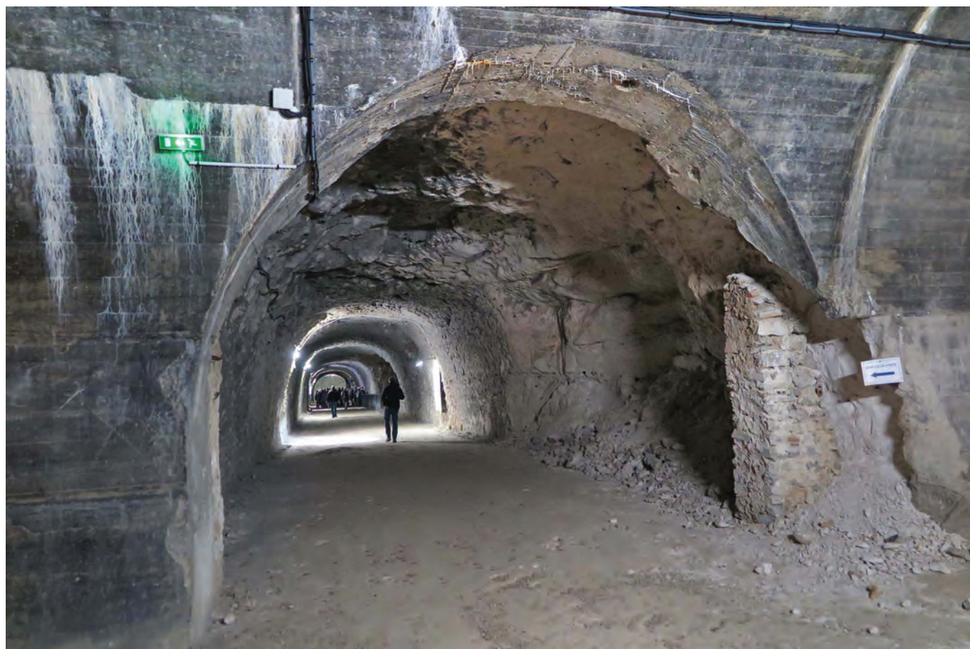
Collapsed roof section off main tunnel at the Mimoyecques V3 site. The Sub Brit party is seen in the distance.
